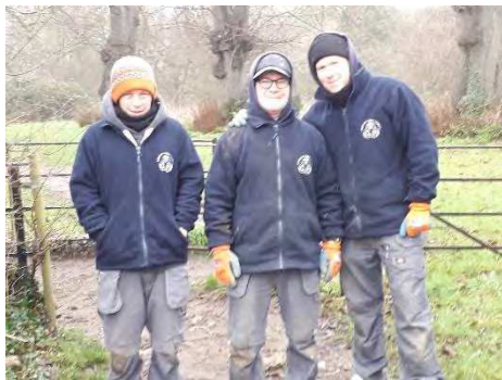
Brad, Gary and Jamie: just finished concreting in the post sockets – bang on target!
